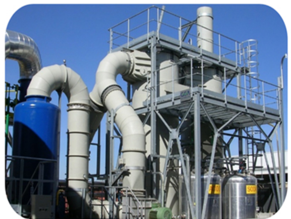
Waste Gas Scrubbing System- SOx NOX & Industrial Gas
